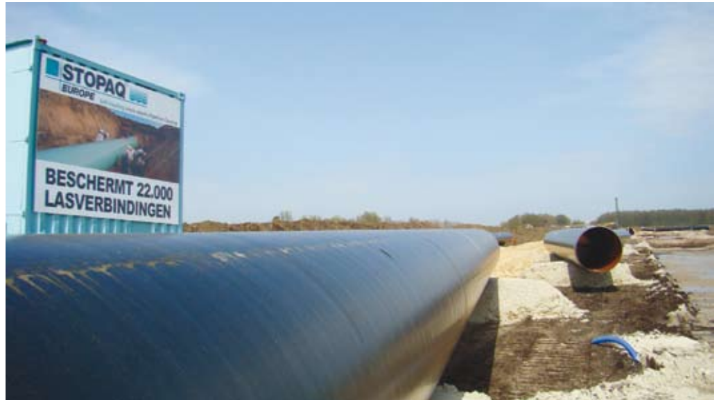
Figure 3. Stopaq containers along the roads in the northern Part of the Netherlands.
